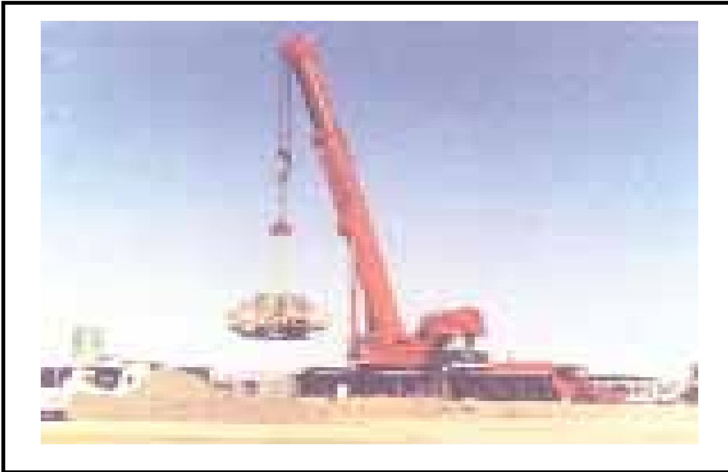
Figure 5b: Single lift (106 tons) of 7.1mø raise bore reamer from shaft within 12 hrs of holing.
